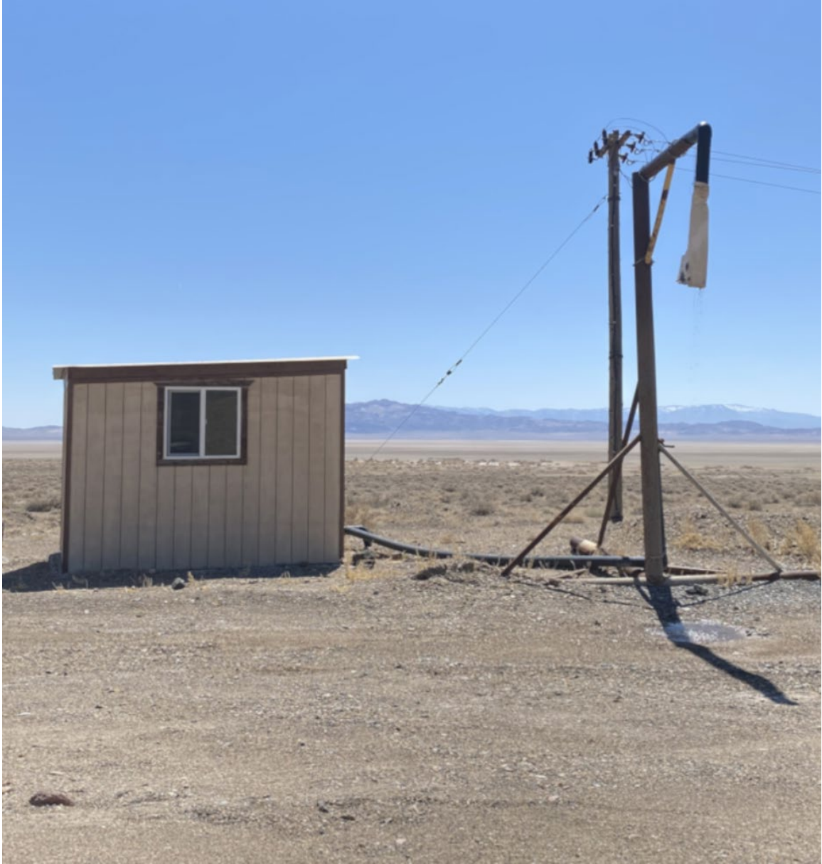
Figure 9 - Photo of the Columbus Marsh site looking south on April 3 rd , 2021. Water is pumped from the shed, and is fed through the depot outlet to the right.
