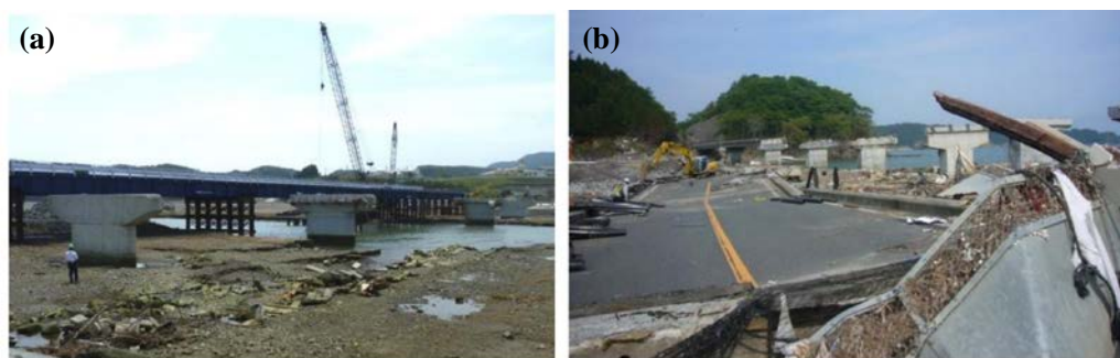
Figure 1. Damaged bridges after the 2011 Great East Japan Earthquake: (a) Koizumi bridge on the left (photo: E. Monzon) and (b) Utatsu Bridge on the right (photo: I. G. Buckle).
