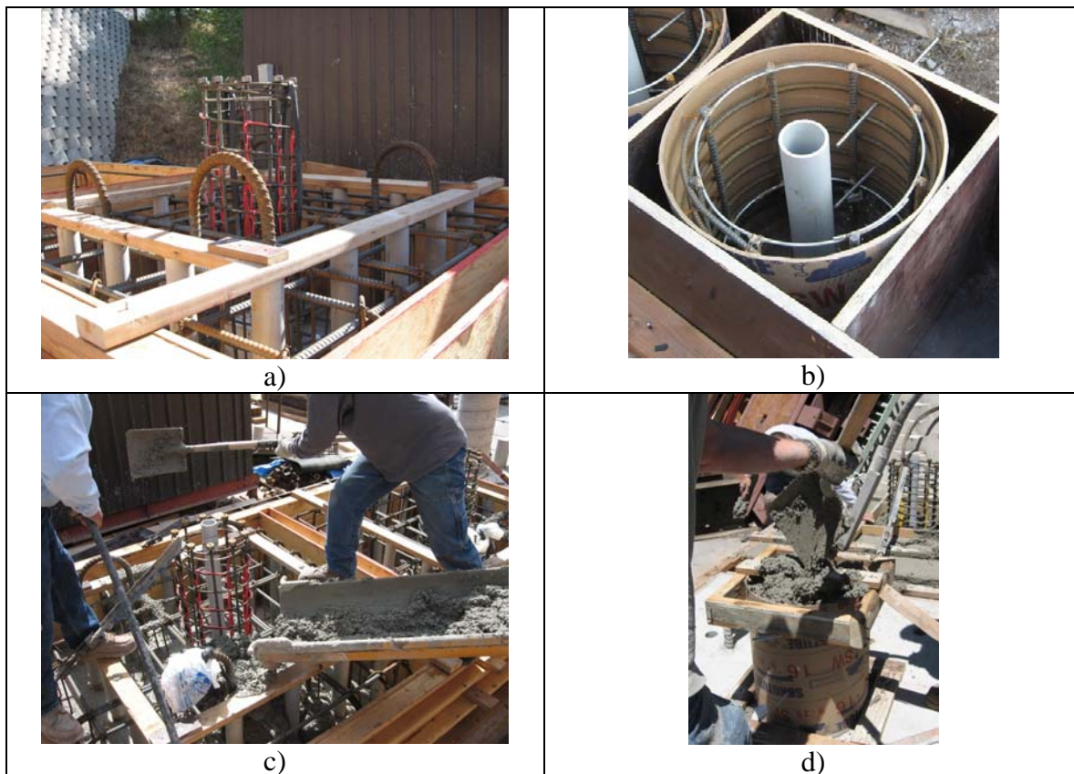
Fig. 2-17. a) Base Segment before Concrete Casting, b) Typical Segment Cage, c) Casting the Footing, d) Casting the Base Segment
