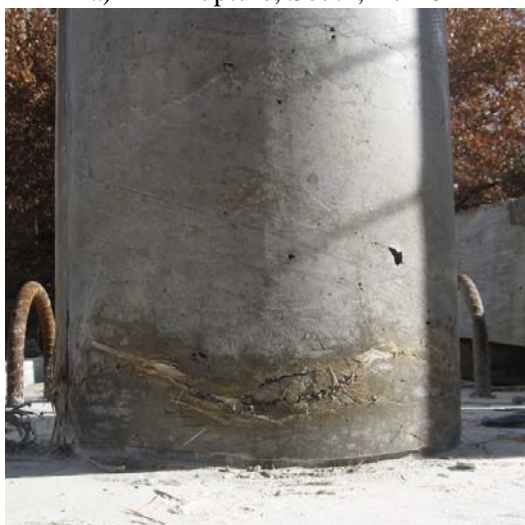
c) Horizontal Crack, South, Run 6
