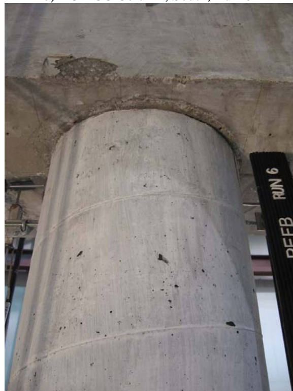
d) RC-ECC Column, West, Run-6
