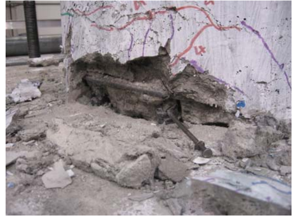
b) RC-ECC Column, South, Run-6
