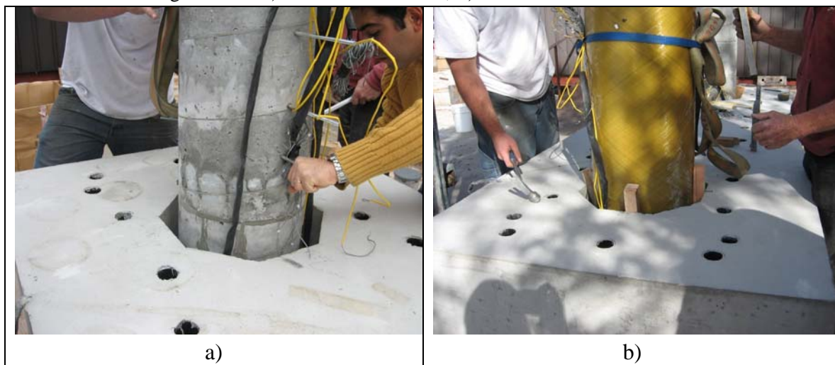
Fig. 2-75. Inserting the Columns in to the Footing a) RC-ECC Column, b) FRP Tube
