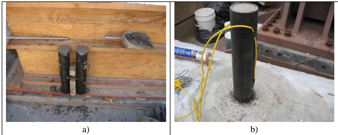
Fig. 2-68. Steel Pipe-Pin, a) Filled with Concrete, b) Sat on the Cap Beam
