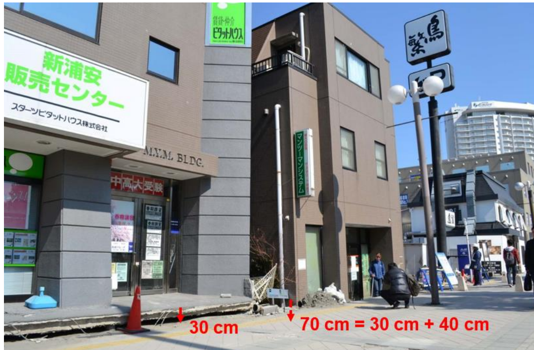
Figure 2-2: Liquefaction-Induced Building Settlement in Uraysu, Japan (Ashford et al. 2011 and Bray 2016)
