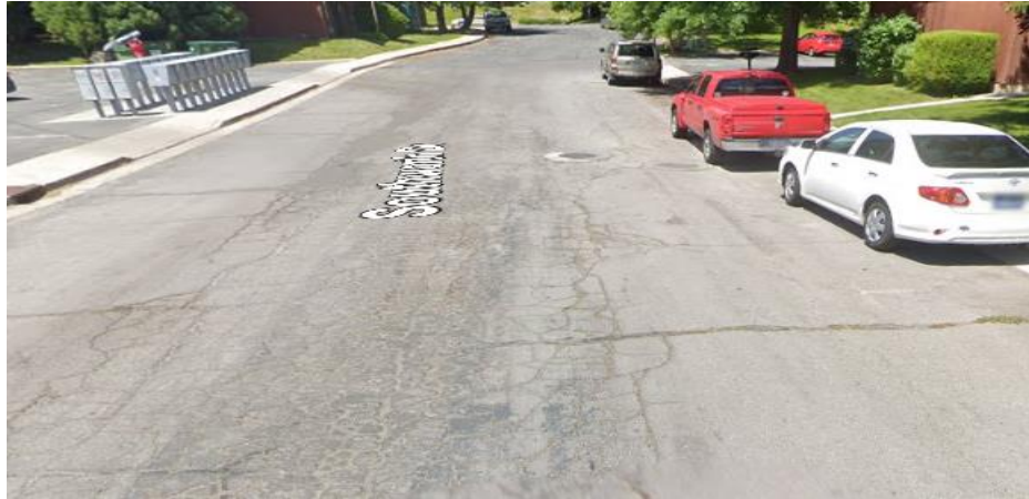
Figure 3. Fatigue Cracking in Asphalt (google earth)
